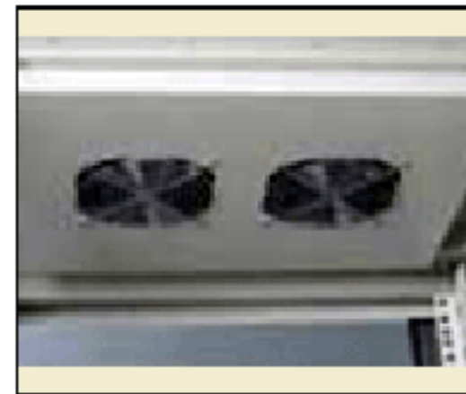
·Cabinets Are Vented To Allow Cooling
